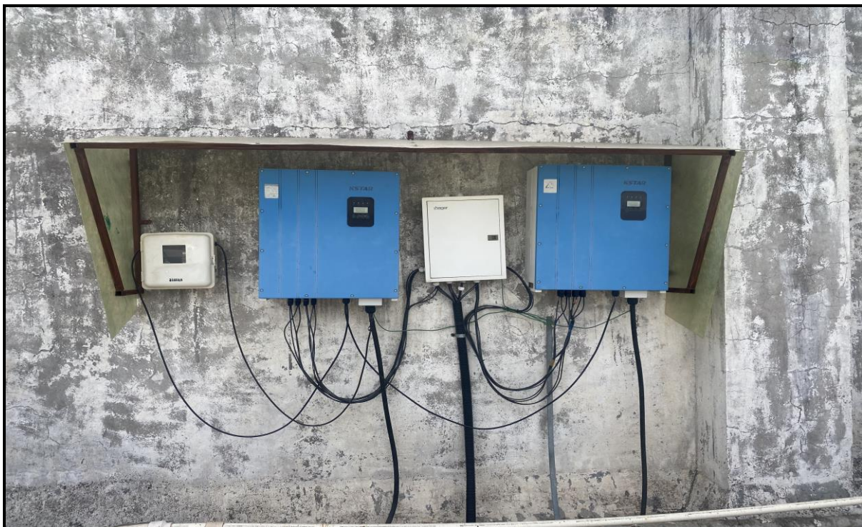
Figure 3.1:- Solar plant 480 KWp and Inverter System
